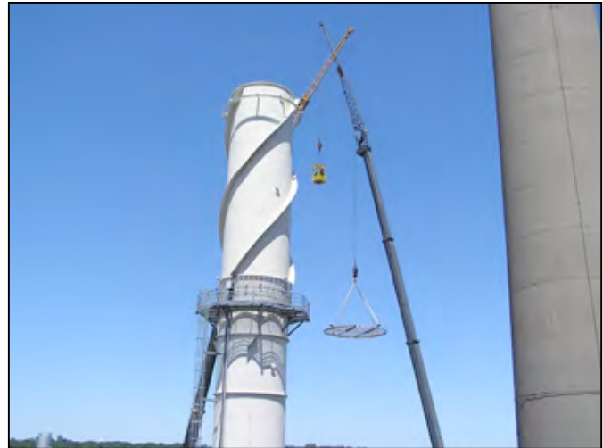
Installing the screen. The small yellow 'box' contains two men who will weld the screen (at right) once it is placed on the top.
